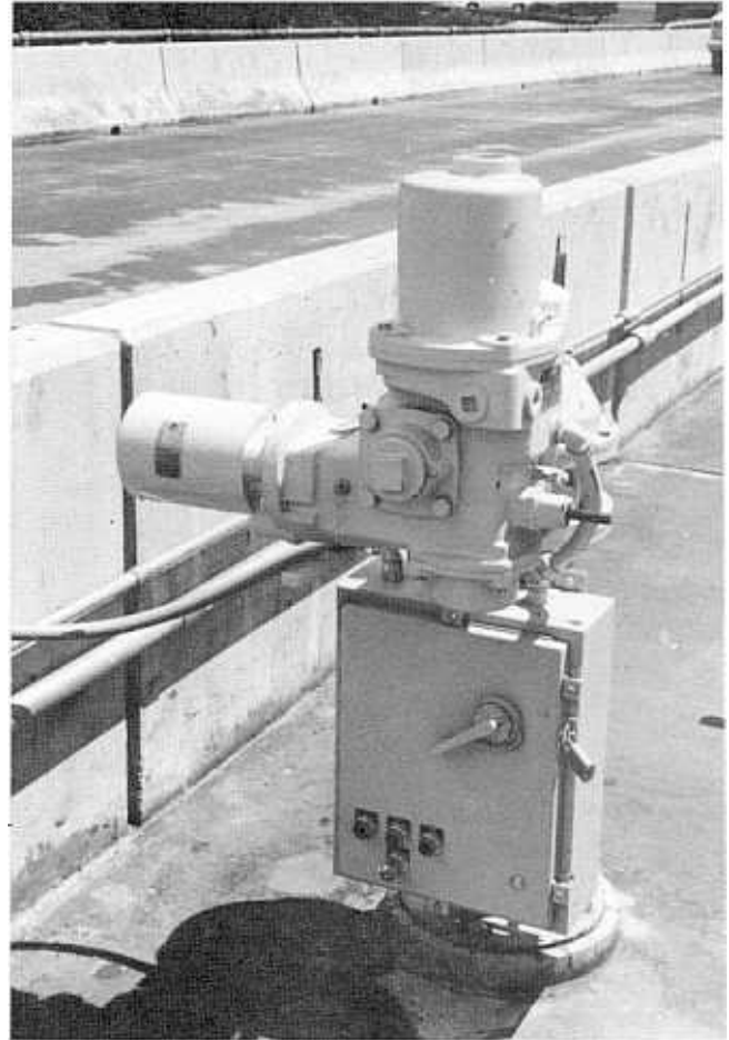
Figure 10-3.—Slide gate motor-operated lift.
