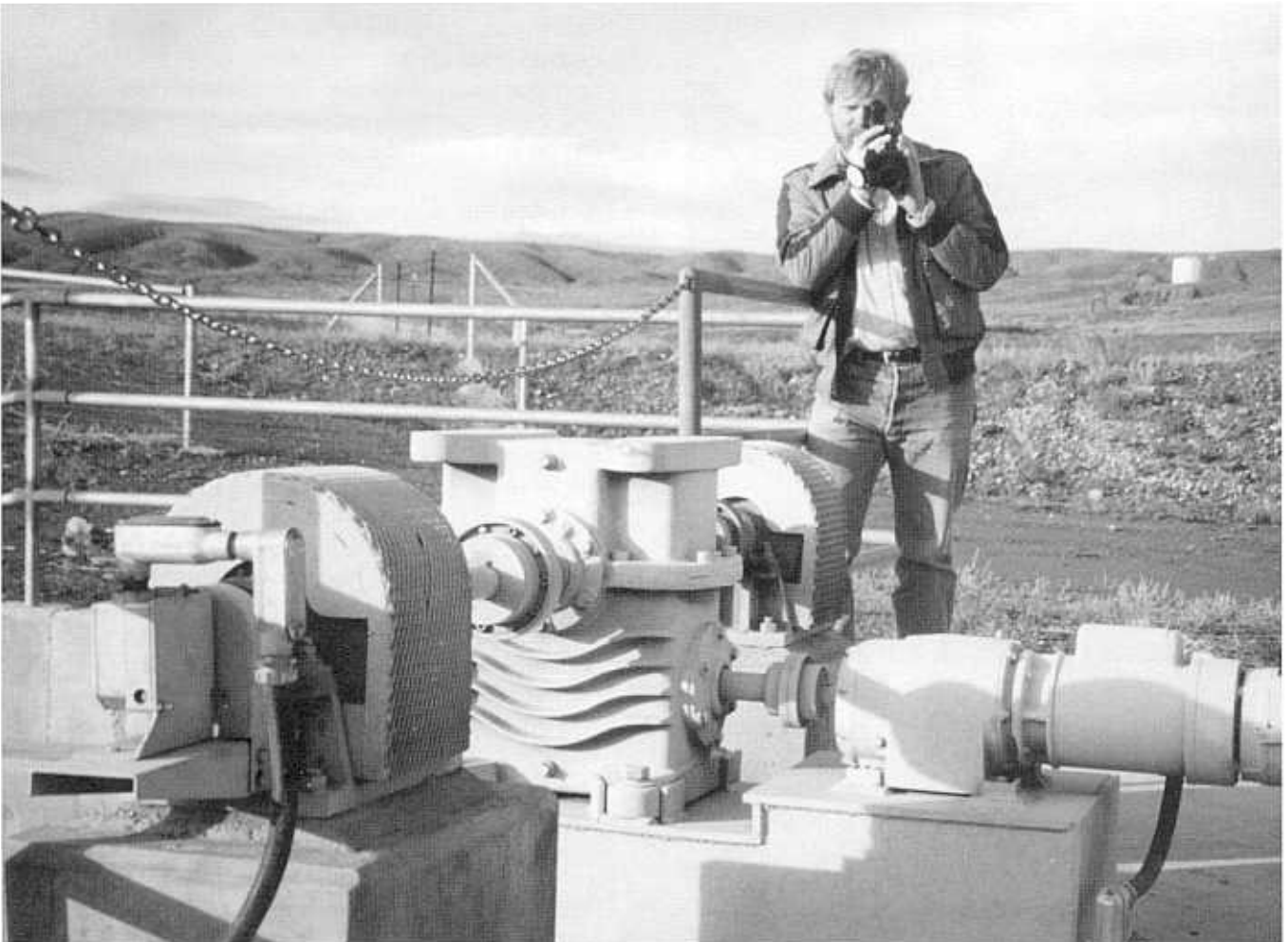
Figure 9-10.—Radial gate hoist with sensor.
