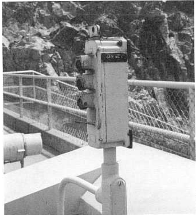
Figure 10-8.—Gate pushbutton controls.
