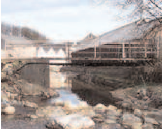
Figure 5: Abutment extends into channel, causing erosion of the left bank (photo courtesy of Royal Haskoning)
