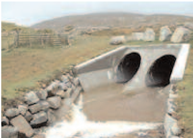
Figure 4: Perched culvert creating a barrier to fish passage
