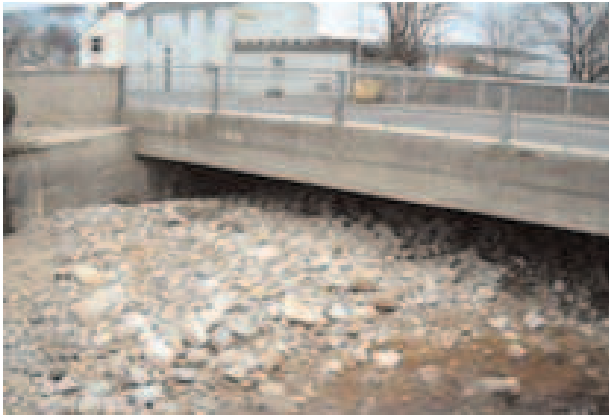
Figure 6: Increased deposition at a bridge
