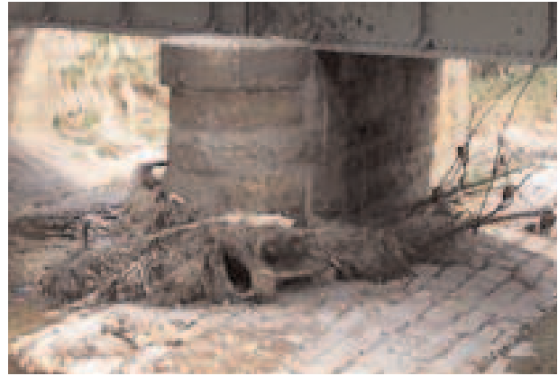
Figure 7: Large woody debris trapped at a bridge (photo courtesy of Royal Haskoning)
