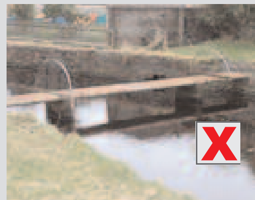
Figure 31 Pipeline/cable laid in channel at risk during high flows
