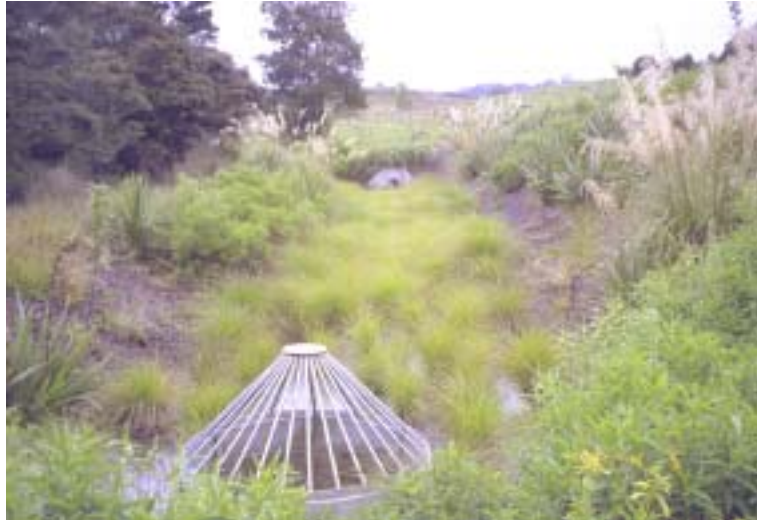
Plate 14-2: Stormwater management pond with significant landscaping
