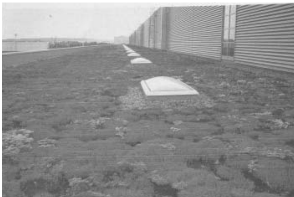
Plate 12-3: Close up view of varied vegetation on a greenroof
