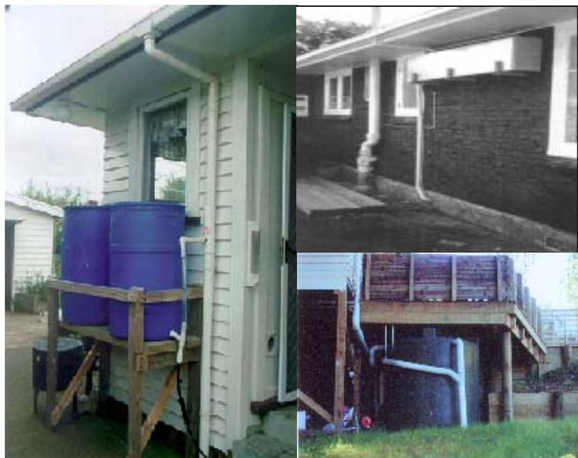
Plate 11-2: Different types of rainwater tanks
