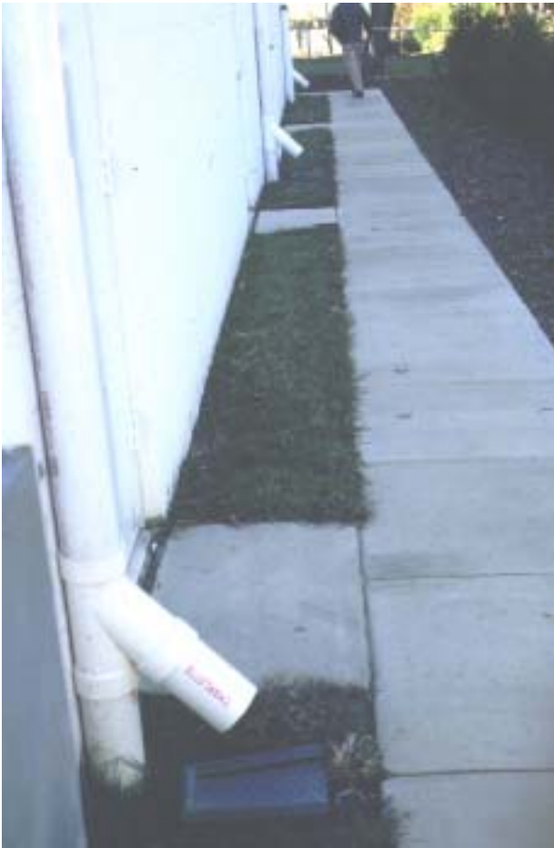
Plate 8-4: Infiltration dry well
