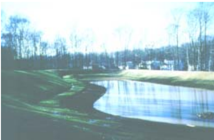
Plate 5-2: Example of a safety bench (above water) in conjunction with a shallow bench (note: normal pool level has been lowered to allow for planting of shallow bench)
