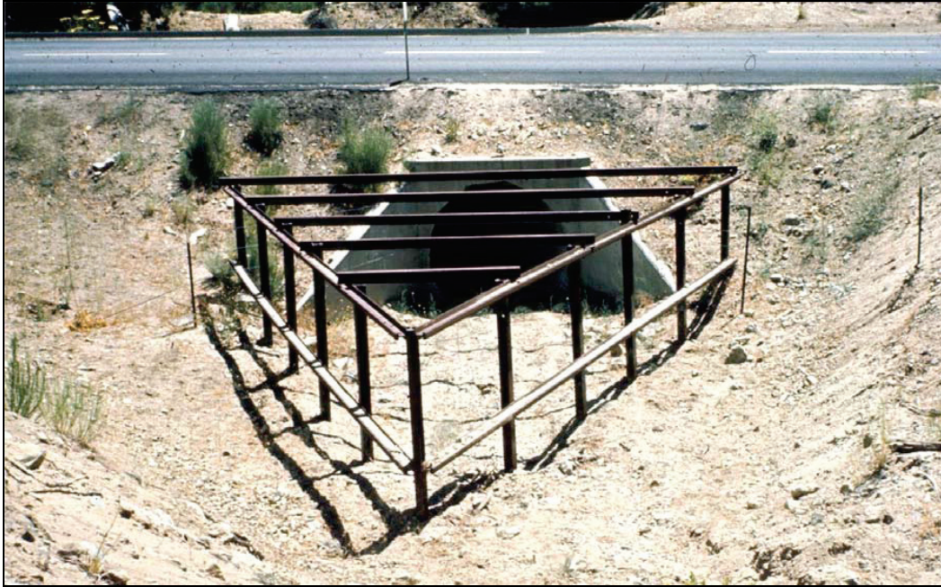
Figure 2.6. Steel rail debris deflector (looking downstream).
