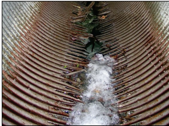
Figure 2.12b. Corrosion issues in a culvert.
