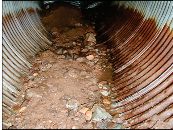
Figure 2.12a. Abrasion issues in a culvert.
