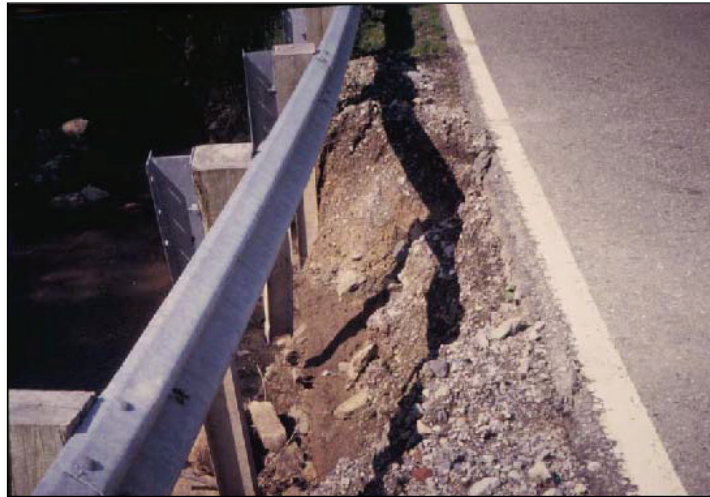
Figure 6.7. Erosion damage to downstream embankment slope from overtopping.
