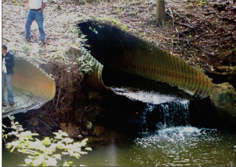
Figure 5.10. Scour at culvert outlet.
