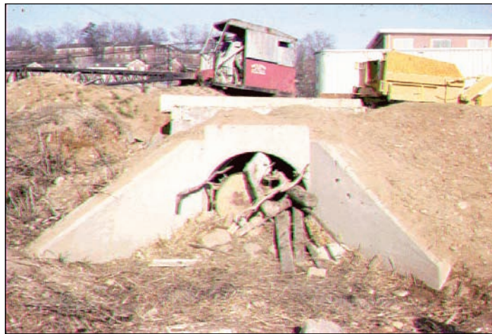
Figure 6.3. Severe debris blockage.
