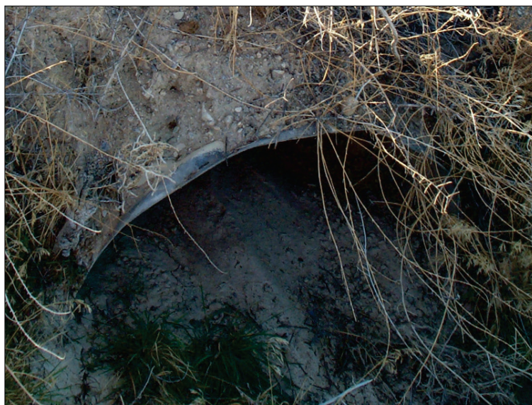
Figure 5.12. Excessive sediment deposition in culvert.
