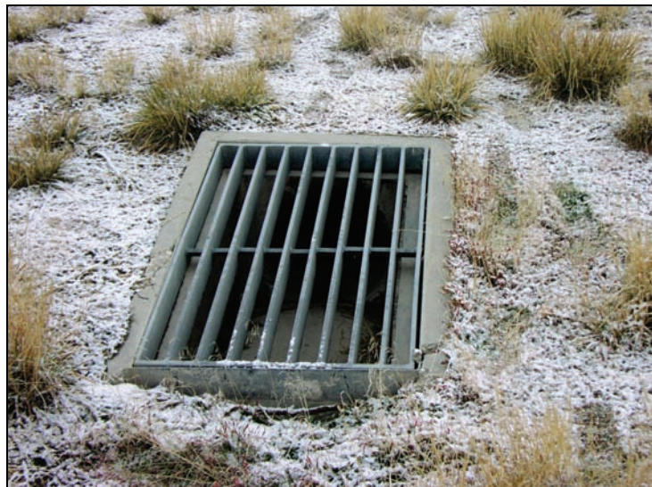
Figure 2.11. Traversable safety grate with proper open area between bars.
