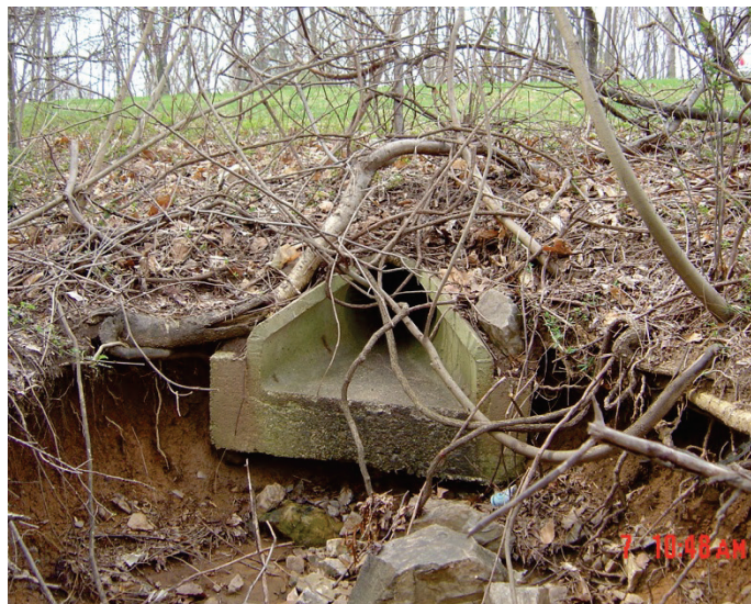
Figure 6.8. Scour hole at outlet of a RCP culvert.
