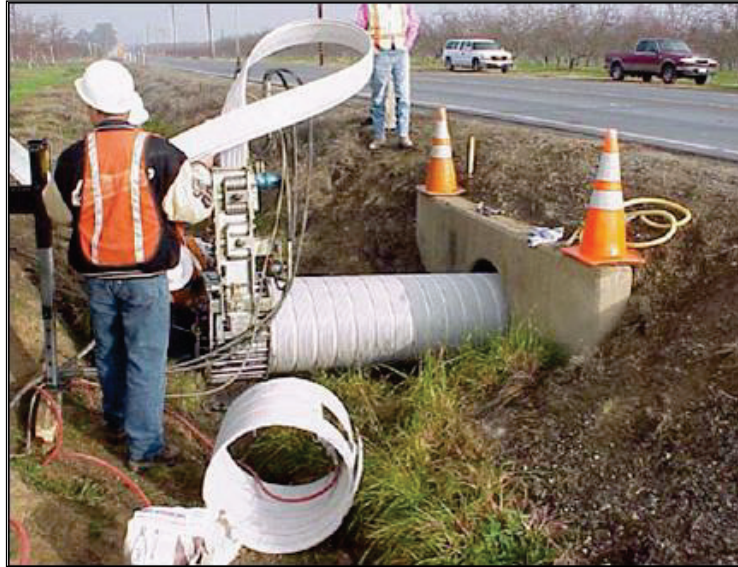
Figure 6.11. Example of a spiral wound liner installation with restricted access at culvert end.
