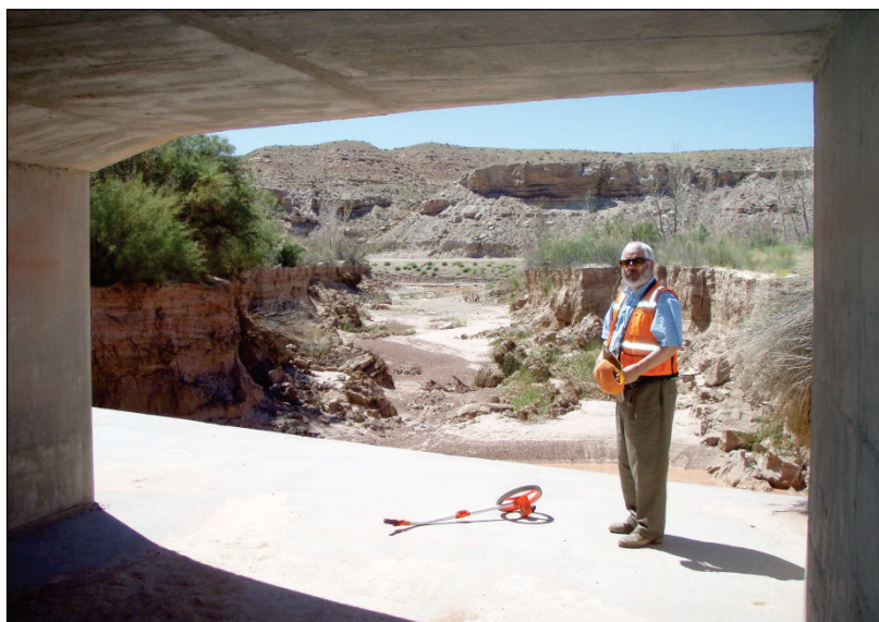
Figure 5.11. Stream degradation downstream of culvert outlet (from Utah DOT).
