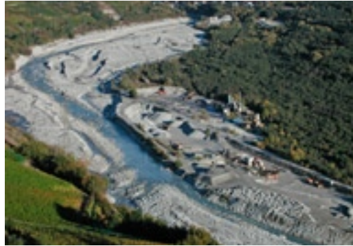
Figure 2.11: Gravel mining in the Rhone River at Pfywald, VS, October 2001 (photo: Eawag).
