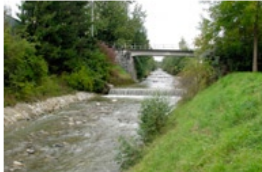
Figure 2.12: Trème: cross-sectional constructions for river bed stabilisation, September 2001 (photo: L. Hunzinger, Schälchli, Abegg + Hunzinger).
