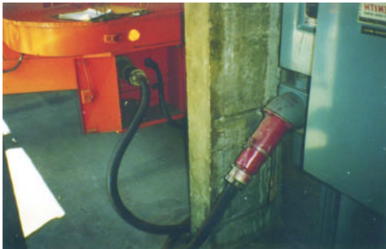
Figure 11-5. Mobile generator and standby power receptacle
