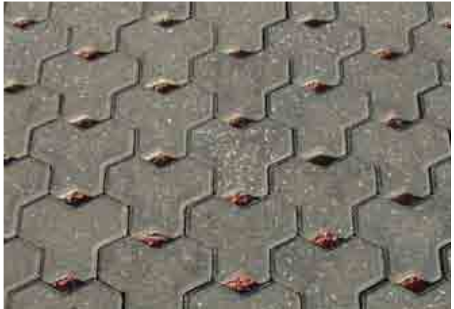
Voids between pavers allow rainwater to trickle through: Bicentennial Park, Sydney, Australia (Credit: Water Sensitive Urban Design)
