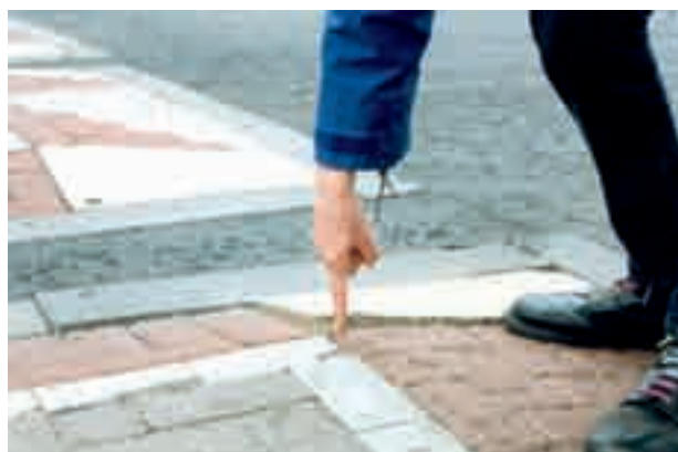
Fig. 2.8 Damage to a speed cushion
