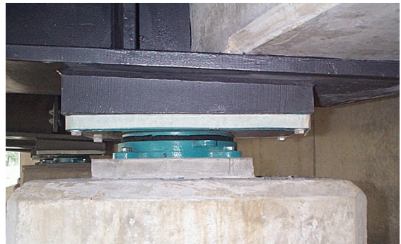
Figure 2 Attachment by bolts in tapped holes (bearing plate is welded to flange)
