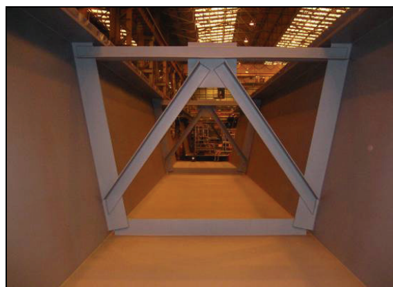
Figure 2 Internal view of a steel box girder where longitudinal stiffeners were avoided by the use of thicker plates
