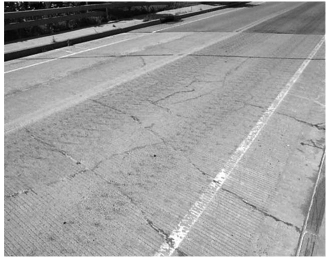
Fig. 1—Methacrylate flood coats are well-suited to concrete slabs that have a large number of random cracks but no evidence of steel corrosion or AAR.
