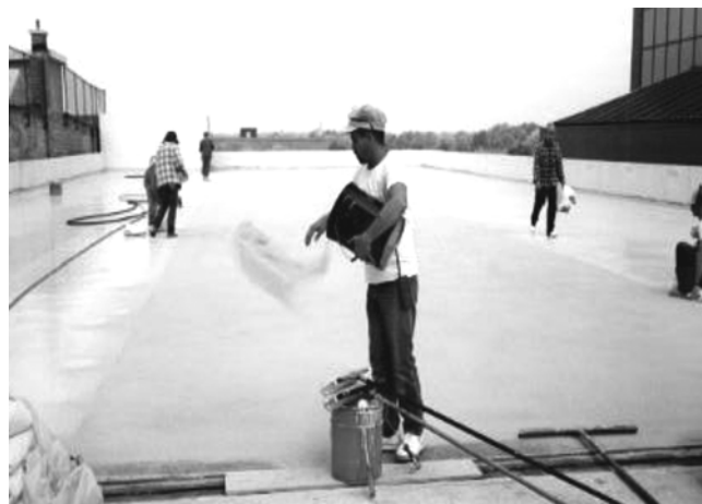
Fig. 3—Aggregate broadcast onto the surface before the resin cures can increase traction.
