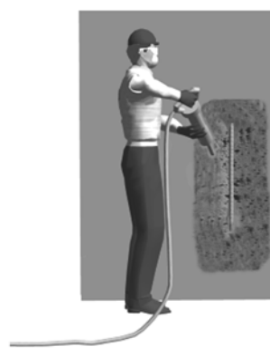
Unsound concrete removed with 15-lb chipping hammer. Hammers larger than a 15-lb class may cause damage to substrate and reinforcement.
