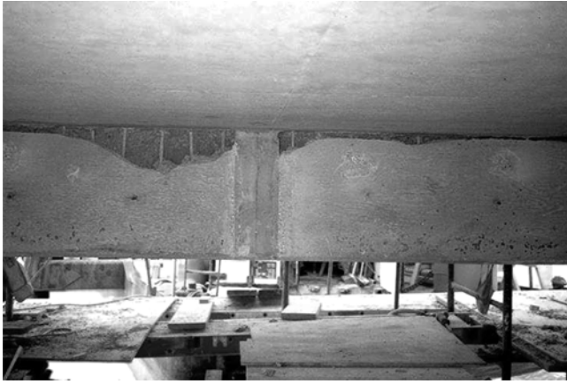
Effects of not filling the cavity.
