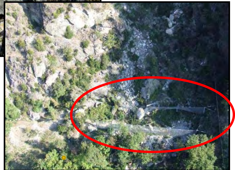
The impacted barrier, Aosta, Oct.. 2009
