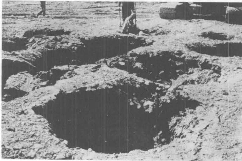
Figure 23. Ground heave induced by dynamic compaction.
