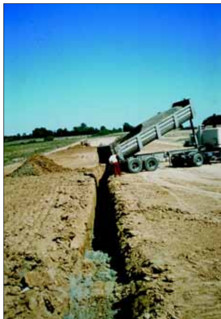
◀ 2 - Vertical drain dug back out of the embankment and filled in with a draining, self-filtering sand (text p. 78).
