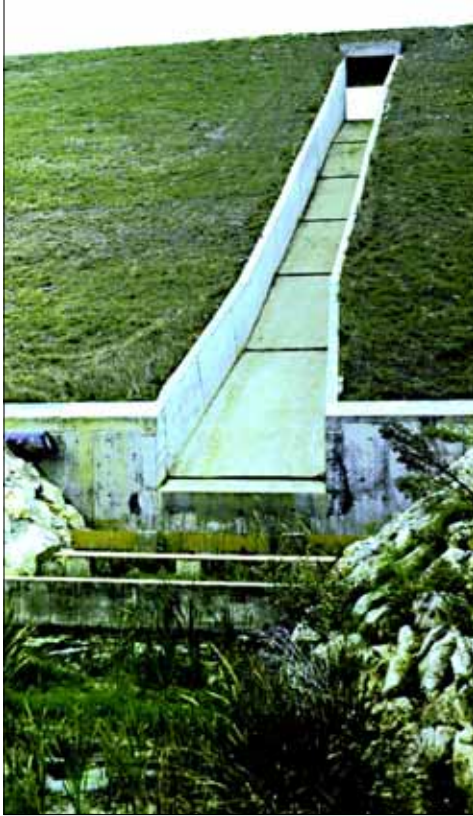
◀ 19 - Frontal inlet spillway, chute set on fill and energy dissipator. (text p.96).
