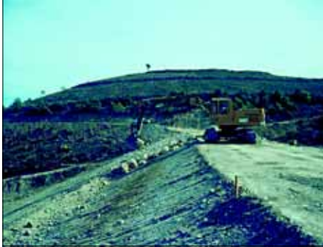
◀ 11 - Placing a rip-rap at the top of a dam with a constant water level. (text p. 76).
