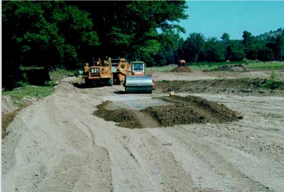
▲ 3 - Test section for a very small dam (at the bottom are the smooth roller compactor and a motor grader conveying earth from the borrow area) (text p. 102).
