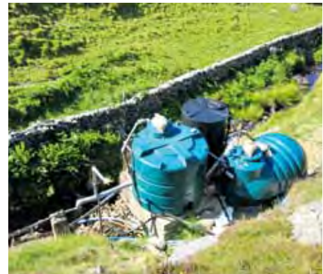
Small community water supply in Scotland. In the European Union, 1 in 10 people (40–50 million people) receive drinking-water from small or very small systems, including private wells (Hulsmann, 2005).
