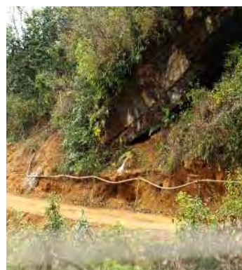
Recent road construction exposed a section of buried mains high-density polyethylene pipeline for a water supply system in Nepal. A vehicle can damage this pipeline (hazardous event), potentially causing disruption of safe water supply to some 70 households (risk).
