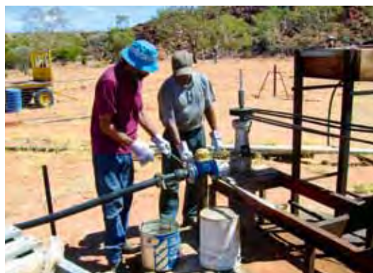
As part of the improvement plan, a water meter is being installed by community members in Australia. Prior to the WSP, the community had no effective means to measure the amount of water they were using.
