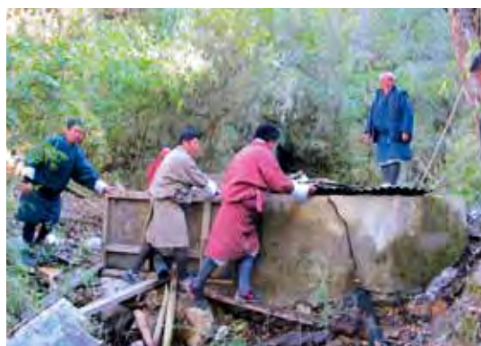
As part of the improvement plan, the damaged wall on an existing intake tank (right) is being repaired, and a supplementary intake tank is under construction (left) in Dhaji, Bhutan
