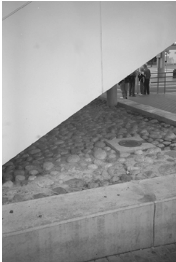
River stone embedded in concrete beneath low overhang discourages vagrancyæBC-Transit, Vancouver, BC Canada
