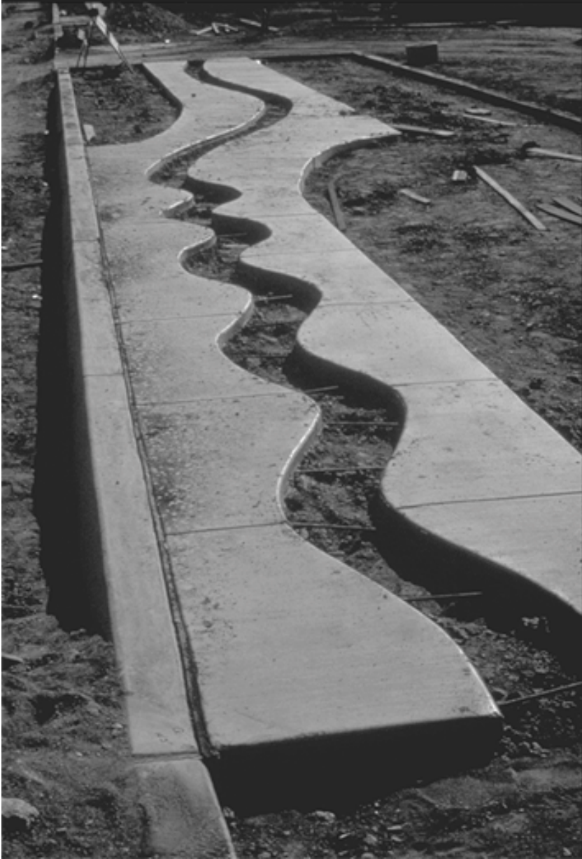
Desert Stream SculptureæTohno Tadi Transit Center and Park-and-Ride, Tucson, Arizona Photo Courtesy of City of Tucson
