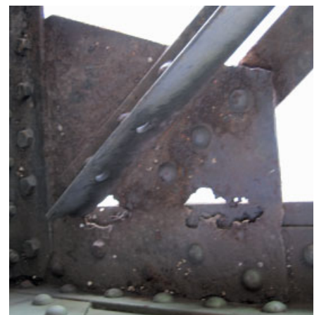
Fig. 9. Severely damaged gusset plate in lower bracing
