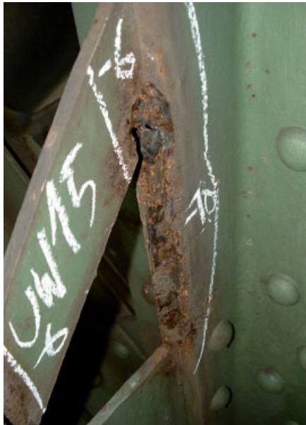
Fig. 10. Corroded area within a strut
