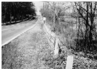
Road Side Hazard Rating 5
